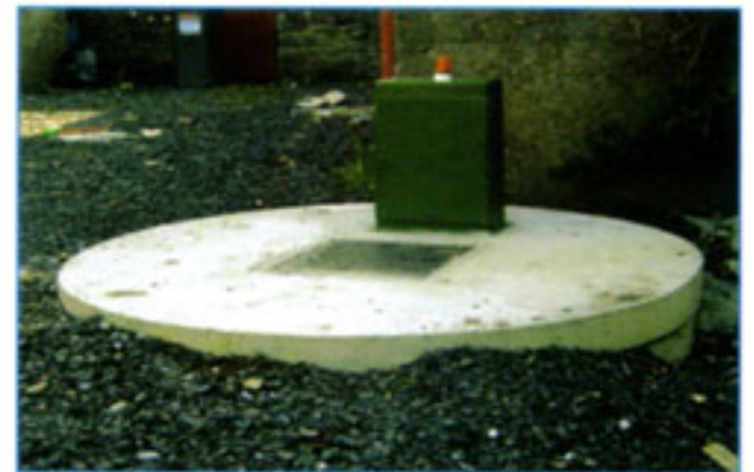
Sewage treatment plant for public house and restaurant
